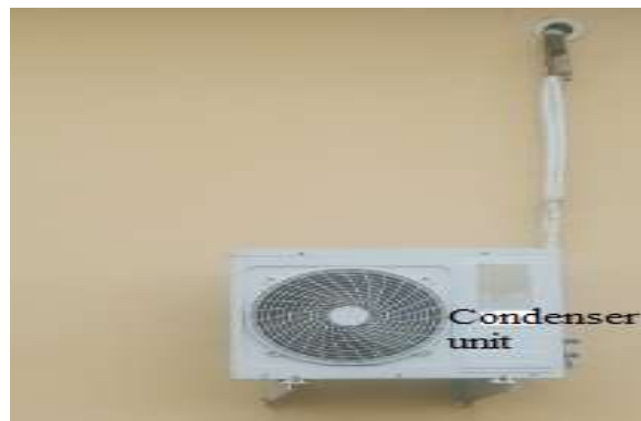
Figure 4: Outside of Central Condensing Unit
